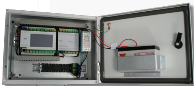
Steel wall casing, open, here with UPS
